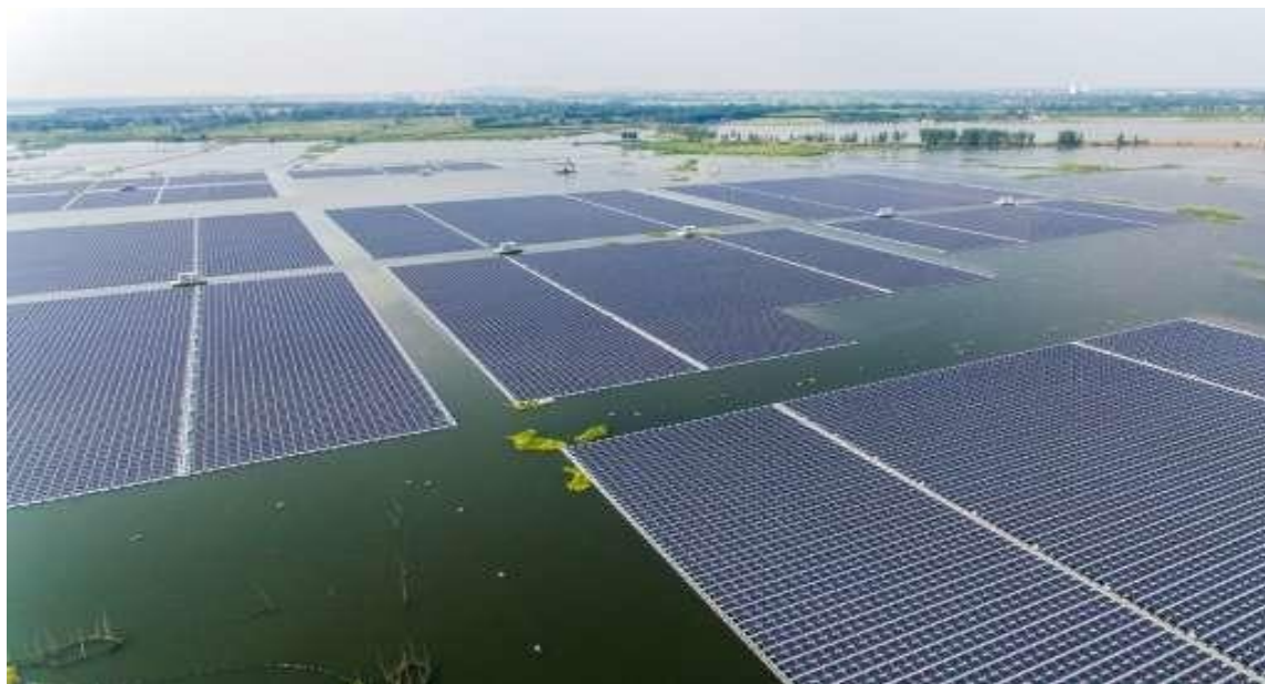
Chandigarh Floating Solar Power Plant, India
