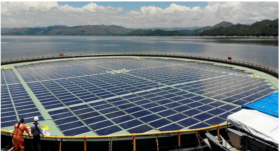
Dezhou Dingzhuang Floating Solar Farm, China
