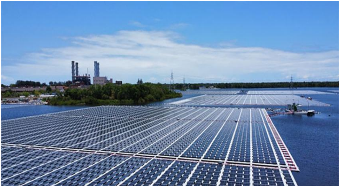
Omkareshwar Floating Solar Power Project, India
