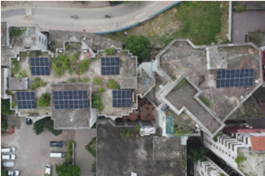
Figure 2 Rooftop Solar System of BIAM Foundation
